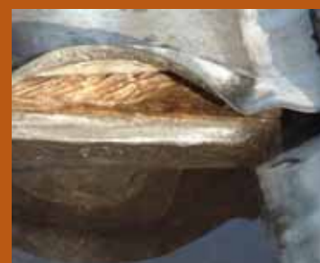
Water penetration: timber decay is often the result
